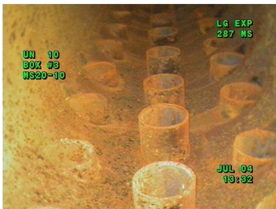
A boroscopic look at rust inside this system
