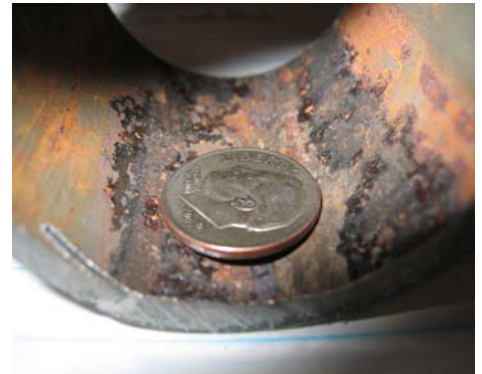
Corrosion and pitting
